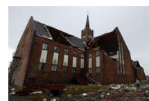
Monday Tornado Damage-2
