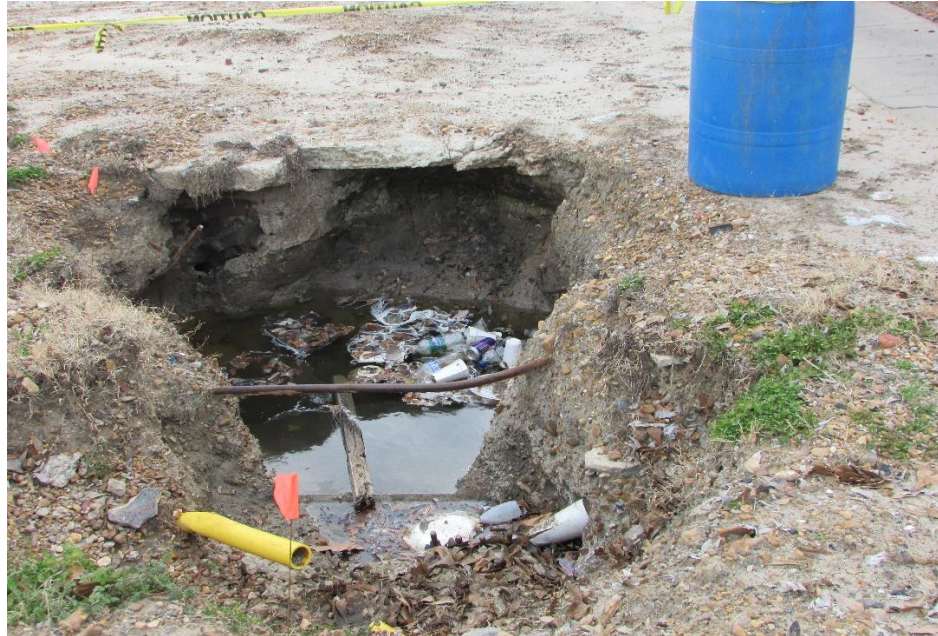
Illustration 4. The break in this water line behind DHH, and the safety hazard presented by the excavation hole are symptomatic of failing infrastructure.
