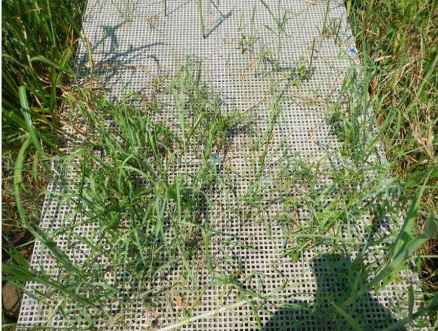
Figure 20: Closer image of grate-decking and vegetation at site HAN-06-A.
