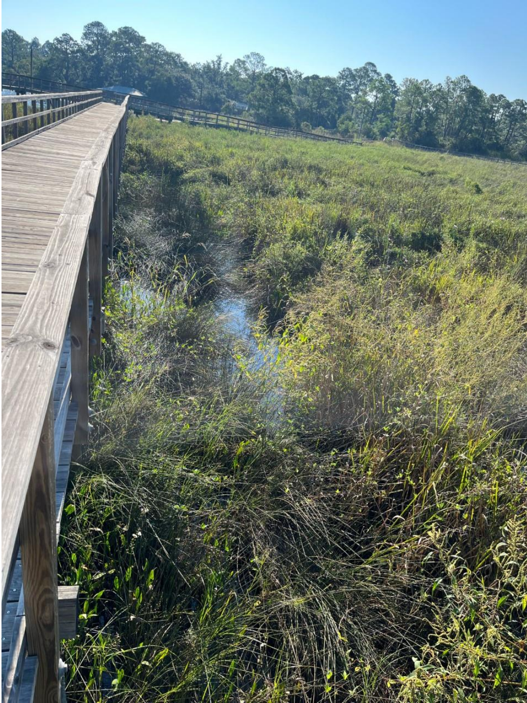
Figure 15: Image of heavy equipment damage at site HAR-05-A in 2021.
