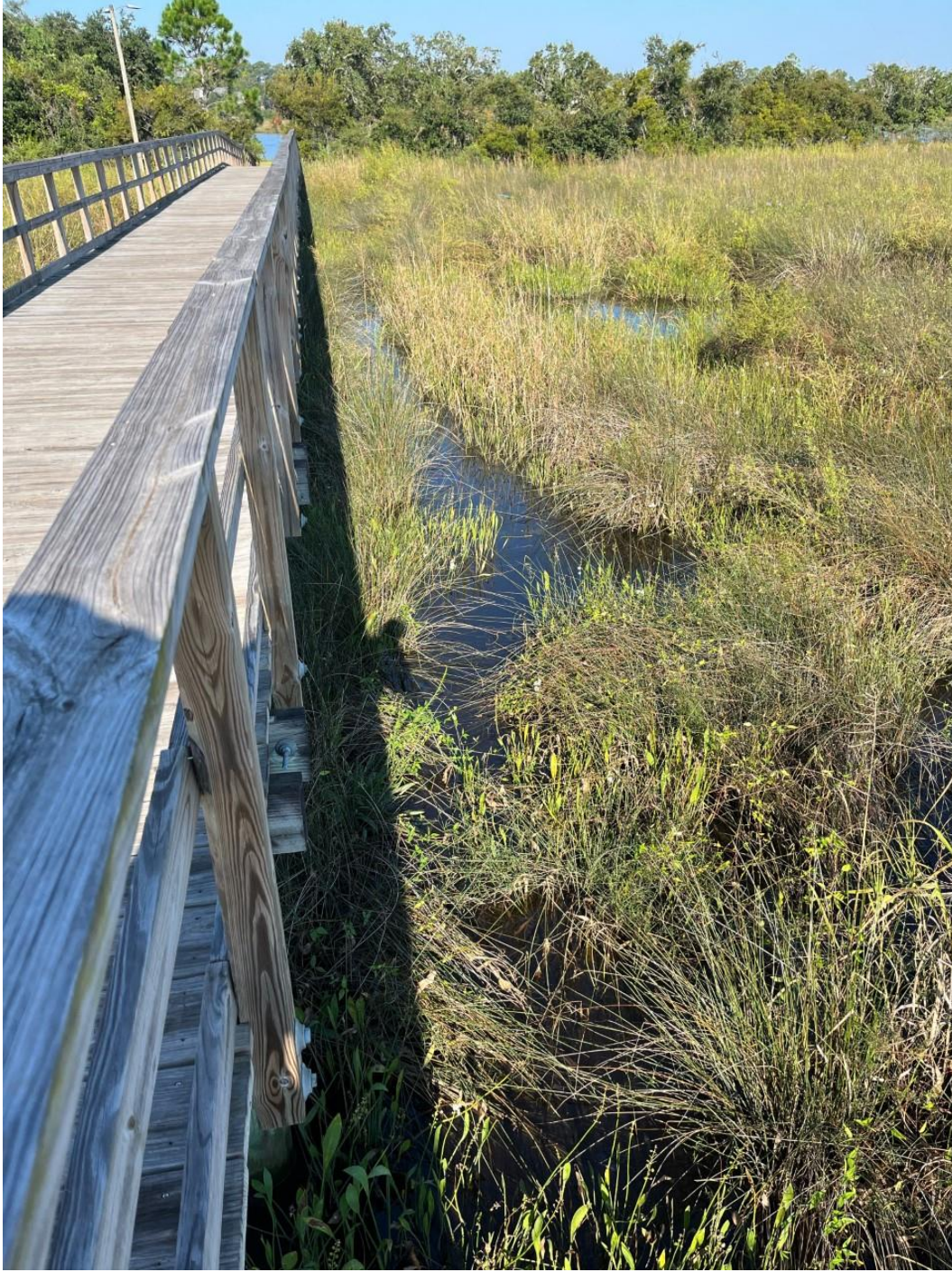
Figure 16: Image of heavy equipment damage at site HAR-05-A in 2021 (opposite side).
