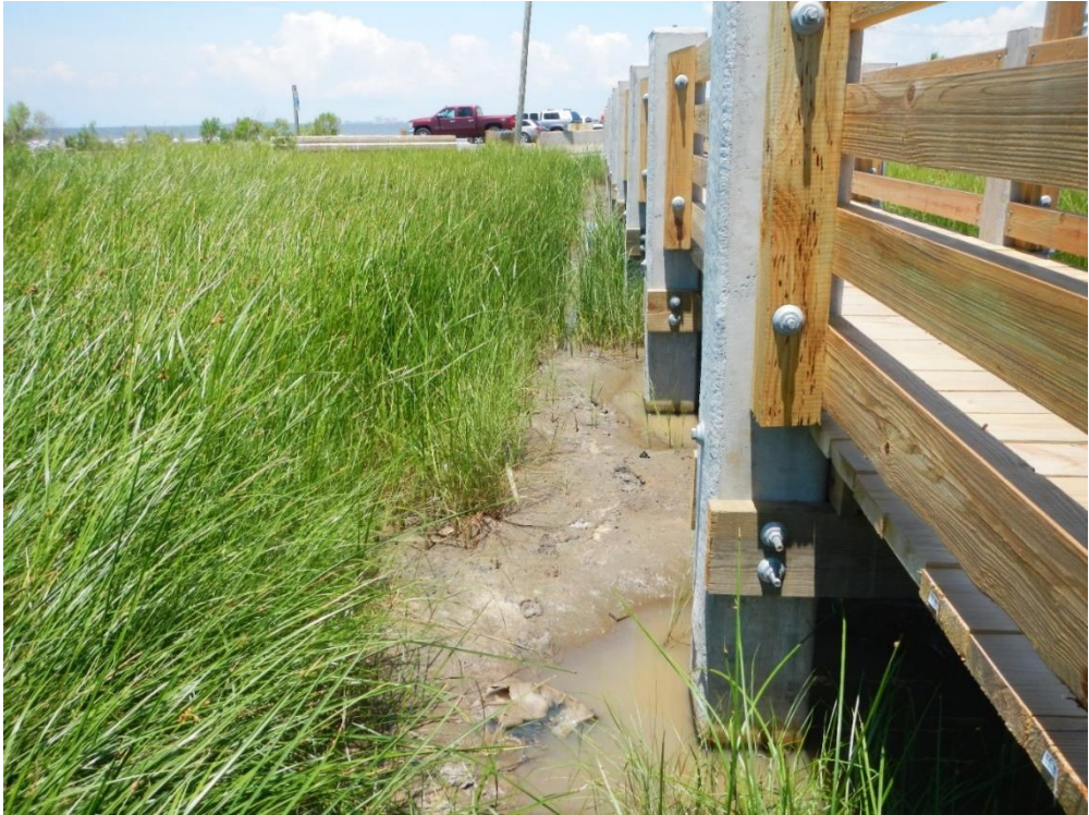
Figure 18: Image of heavy equipment damage from site JAC-12-A in 2021.
