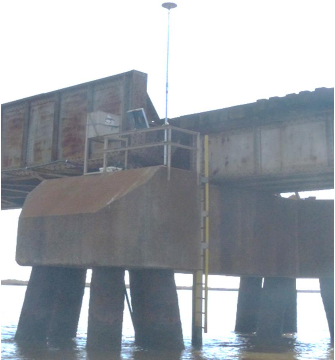
Figure 2.3 GPS setup at CSX RR station.
